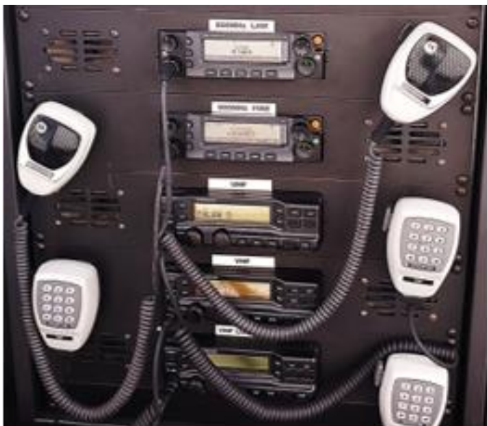
Control 7 radio operator position.
