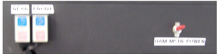
Power switch (right) for turning power off to the radios and antenna mounts.
